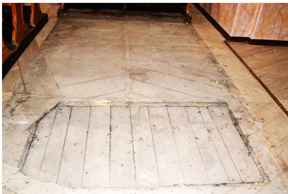
Fig. 8. Szczuczyn. Entrance to the crypt under the benches on the right side of the central nave. Photo M. Majorek.
