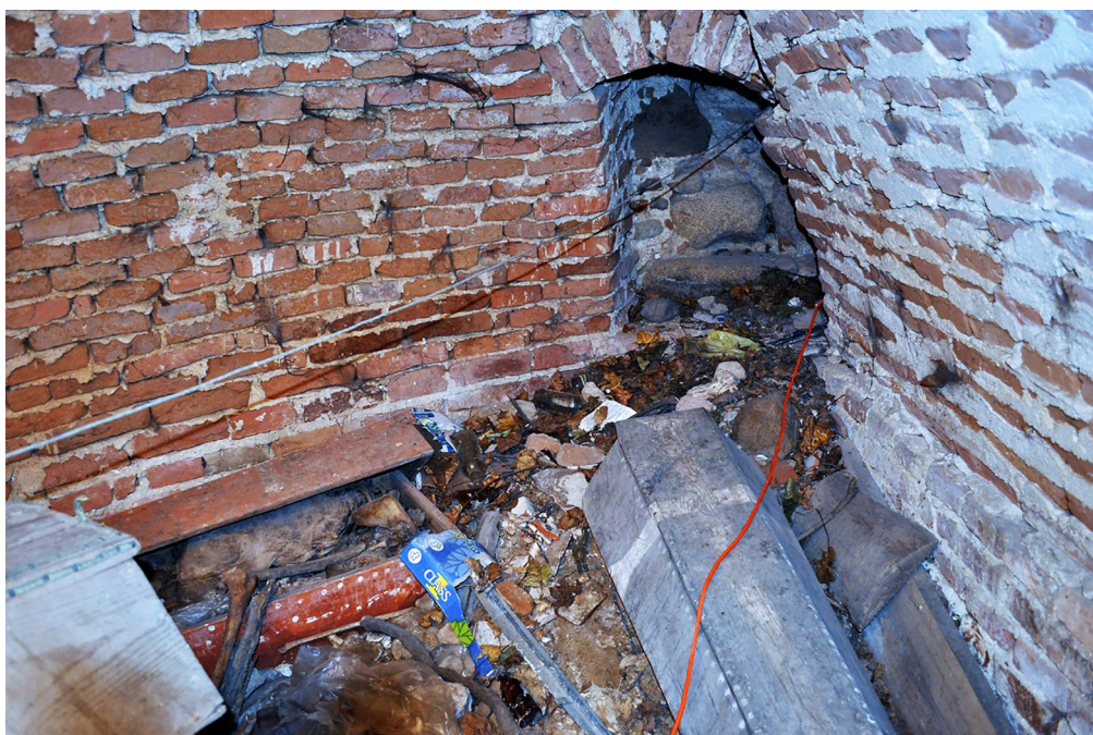
Fig. 7. Szczuczyn. Passage between two crypts connected to the ventilation shaft. Photo M. Nowak.
