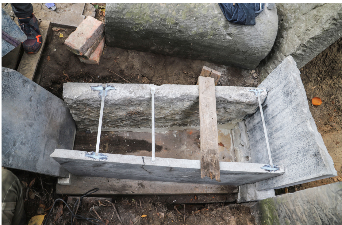
Fig. 4. Warsaw, Wola necropolis. Grave No. 428 – conservation work, visible sandstone foundation supporting stone kerbs on which a half-cylinder slab will be placed. Photo: D. Pisarski.
